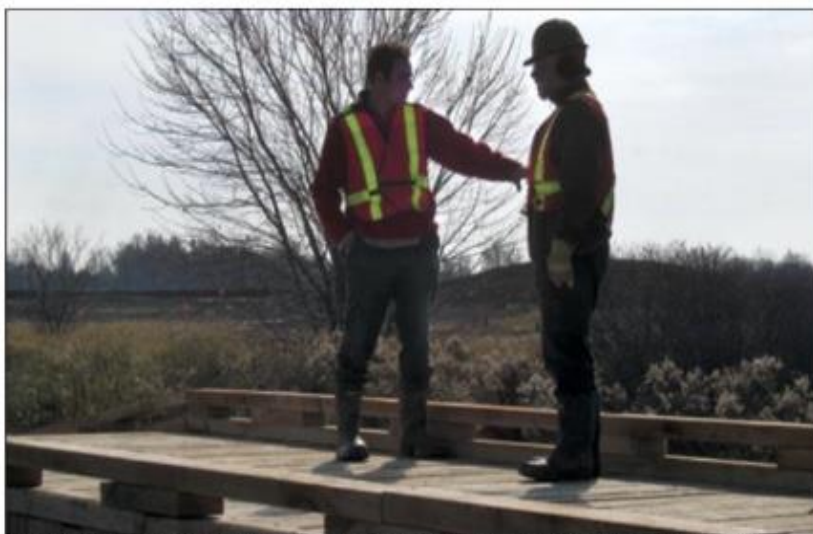
(L-R) Tim Muys and team member on 1 out of 9 oak bridges the team built during construction of Piper's Heath GC.
